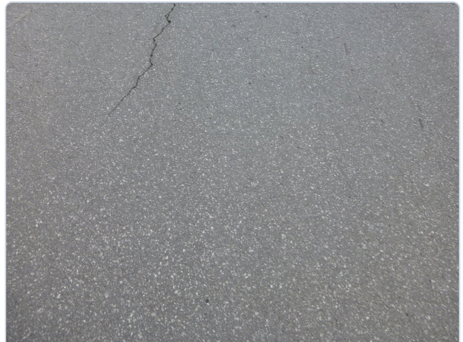
Exhibit S-1. Hairline crack along slab perimeter, west elevation.
