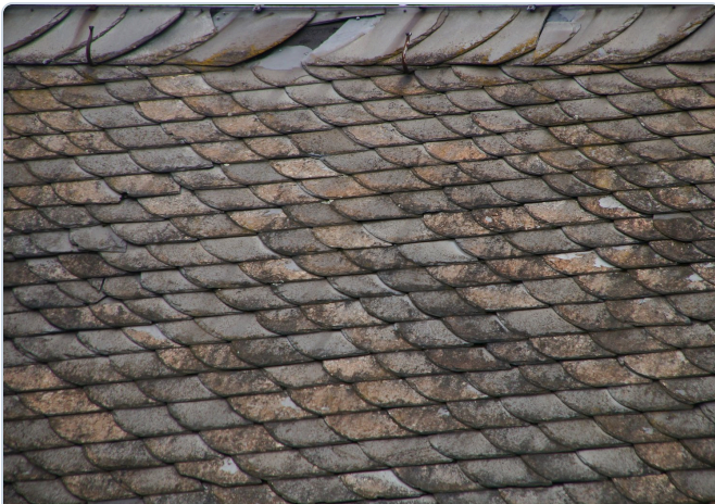
Exhibit R-1. Hail damage on roof shingles, south face.
